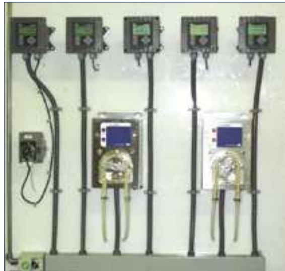
Central control system for 5 stage pretreatment washer controls alkaline cleaner, rinse stages, phosphatizer stage and final seal rinse stage. Chemical feed pumps are included on the panel.
